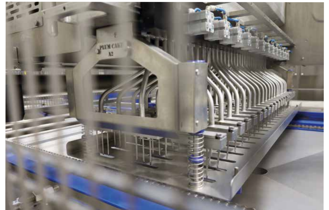
Product cooling tunnel
